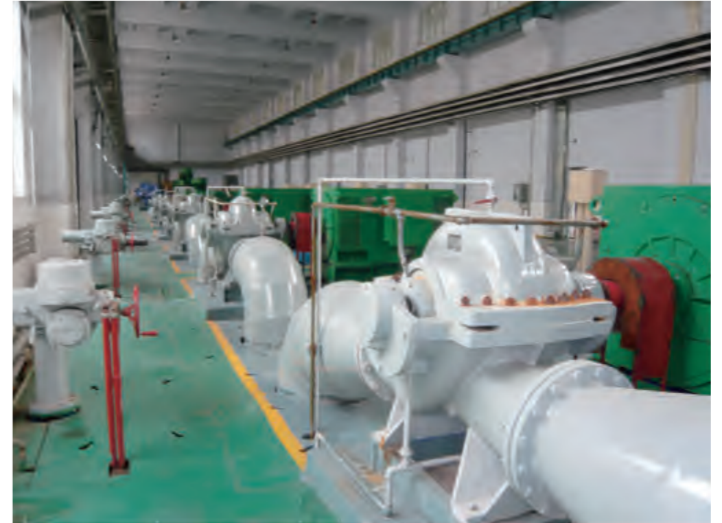
↑ 辽宁鞍钢 Liaoning Anshan Steel (SLOW400-500(I),2台、SLOW,11台)
